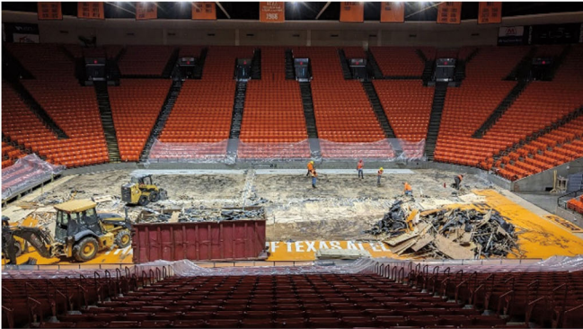
University of Texas at El Paso - Don Haskins Special Events Center Subsurface Improvements
